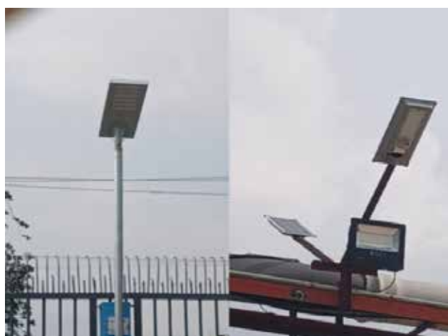
Solar lighting for perimeter fencing.
